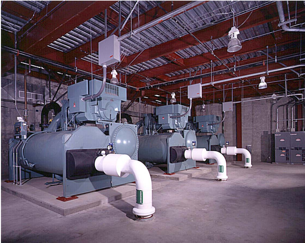
Figure 1-2.1 Typical central plant chiller room with three York electric chillers
