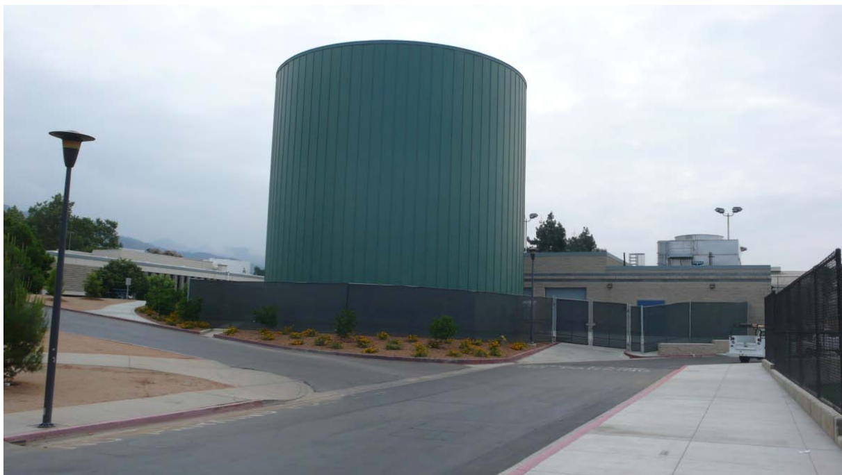
Figure 1-3.1 Typical TES tank on a college campus, this particular one has 7,200-Ton-hrs and is 55ft in diameter and 45ft tall.
