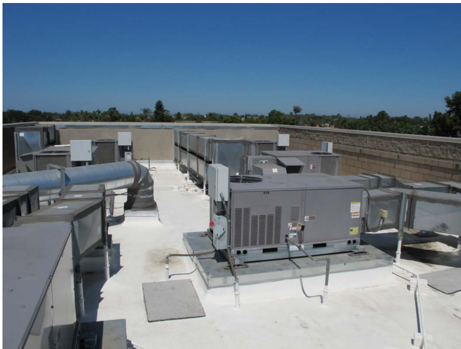
Figure 1-4.7 Typical roof-top AC package units on classroom building
