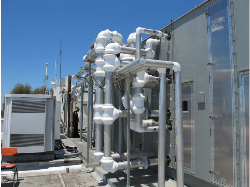
Figure 1-4.2 Dunlap Hall roof-top AC equipment
