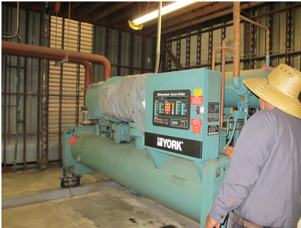
Figure 1-4.9 York water chiller in penthouse mechanical room on Russell Hall
