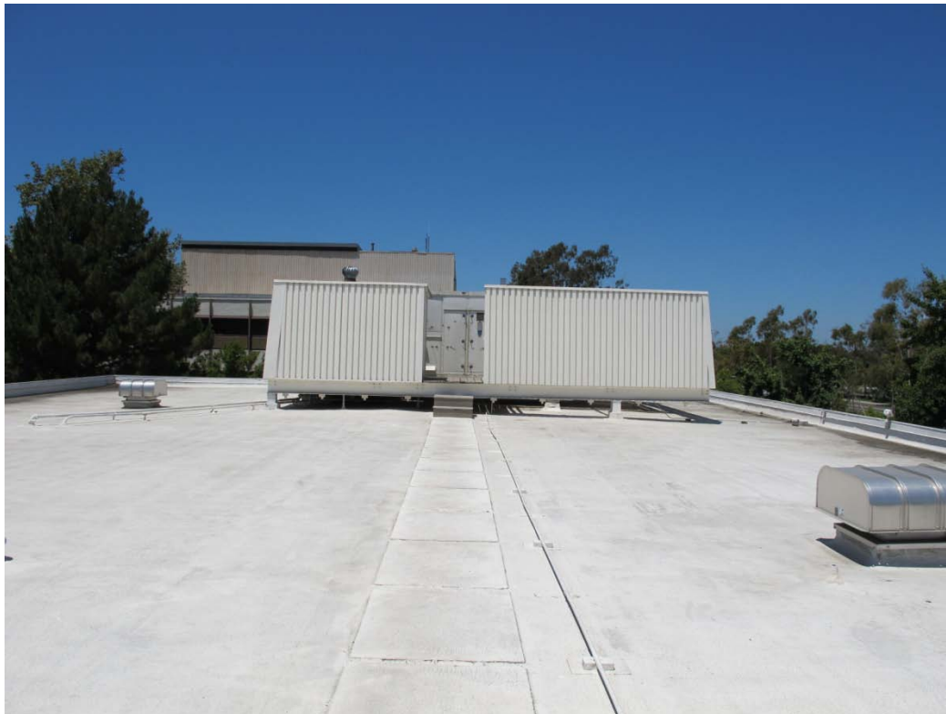
Figure 1-4.10 Screened mechanical equipment on the roof of building "S"
