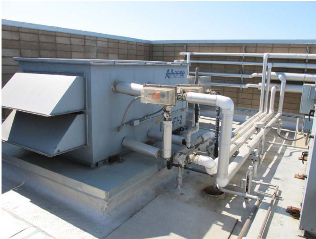
Figure 1-4.4 Typical fan coil unit on the roof of building "F"
