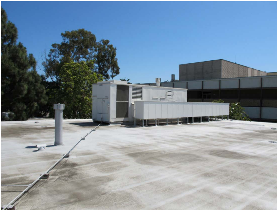
Figure 1-4.11 Multi-zone AC package unit on the roof of Building "T"
