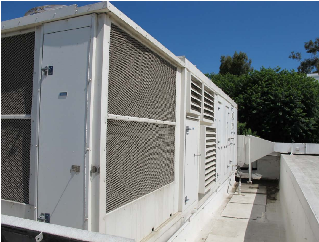
Figure 1-4.12 Roof top multi-zone AC unit on the roof of building "W"
