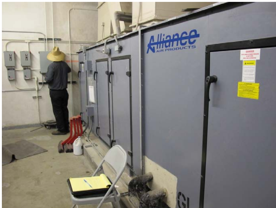
Figure 1-4.5 Cook Gym air handler
