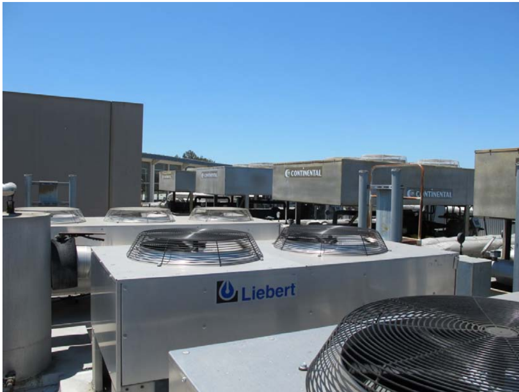
Figure 1-4.1 Roof-top AC equipment on Chavez Hall
