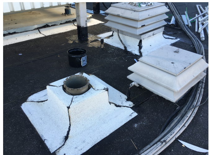
Capsheets and liquid flashings being installed around roof vents and roof penetrations.
