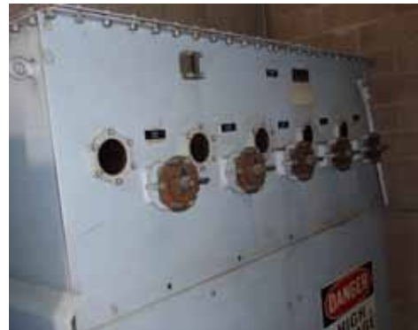
Typical 15KV Selector Switch in Building
