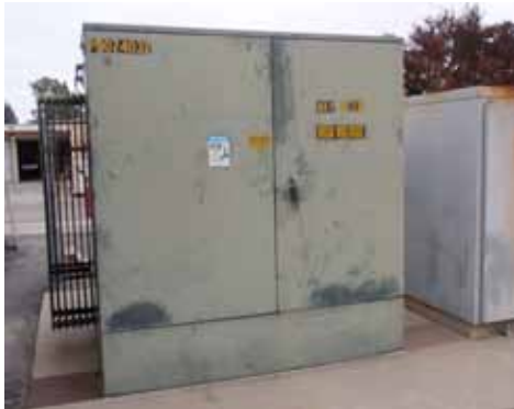
Typical Pad Mount Transformers
