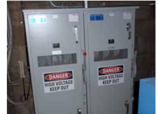
Typical 5-KV Air Switches
